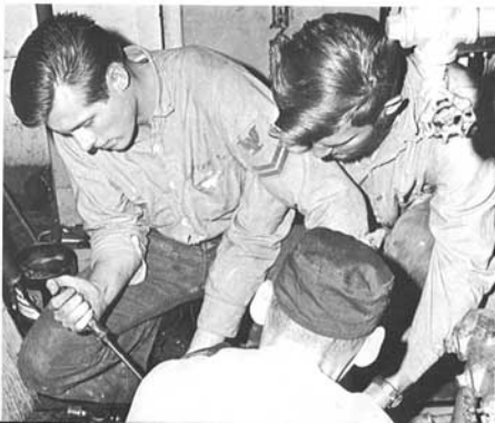
Shaffer, Wilkie and Dykes repair a circulating pump for the boiler. The pump, a primary source of trouble for the BT's forces water through the coils of the boiler.
